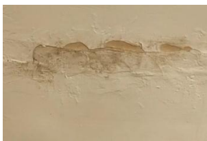
Water damage inside the building
